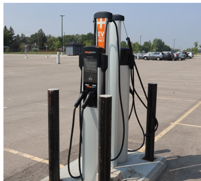
An EV charging station in Niverville.
