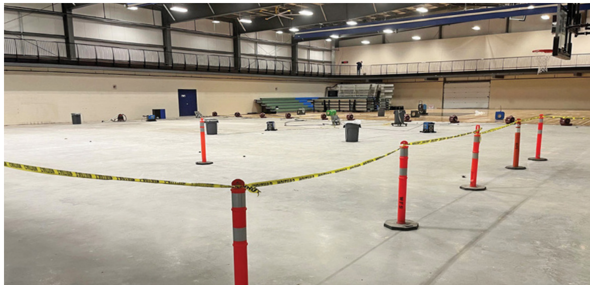
The floor in the CRRC fieldhouse is undergoing repairs.
