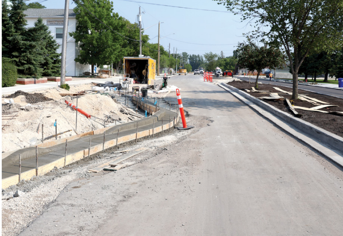
A series of bump-outs are being installed along Main Street in Île-des-Chênes.
