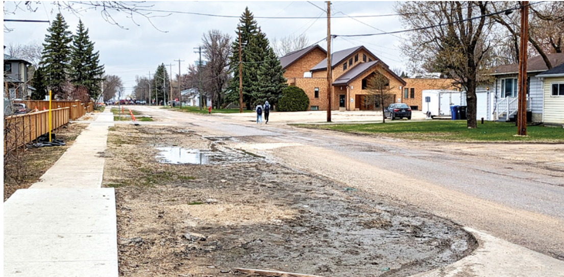
Fourth Avenue South in Niverville is one of many streets to undergo repair work this summer.
